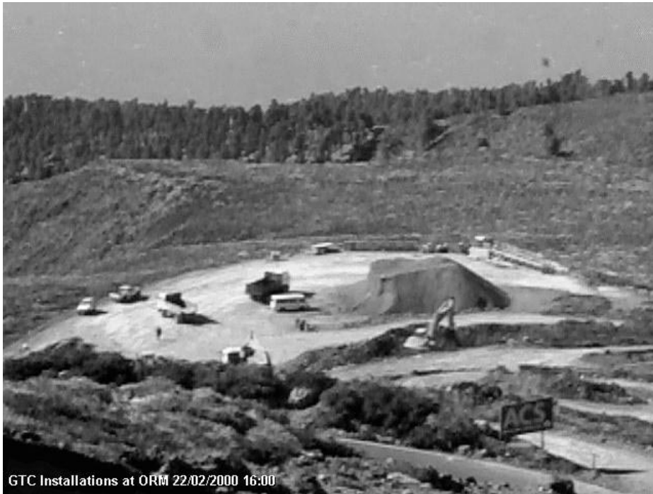
Figure 2.- Web camera view of the work performed at GTC site until the 22/02/00
